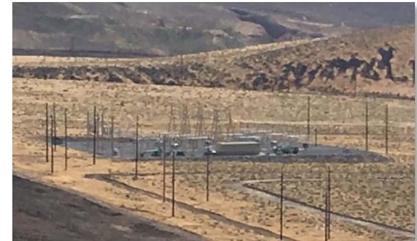
NV Energy's Pah Rah Substation
